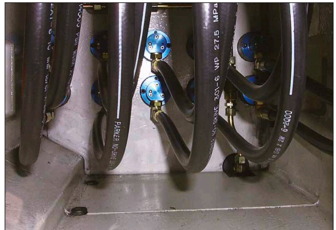
Deublin 1117 Bearingless Unions on Automotive Transfer Line.
